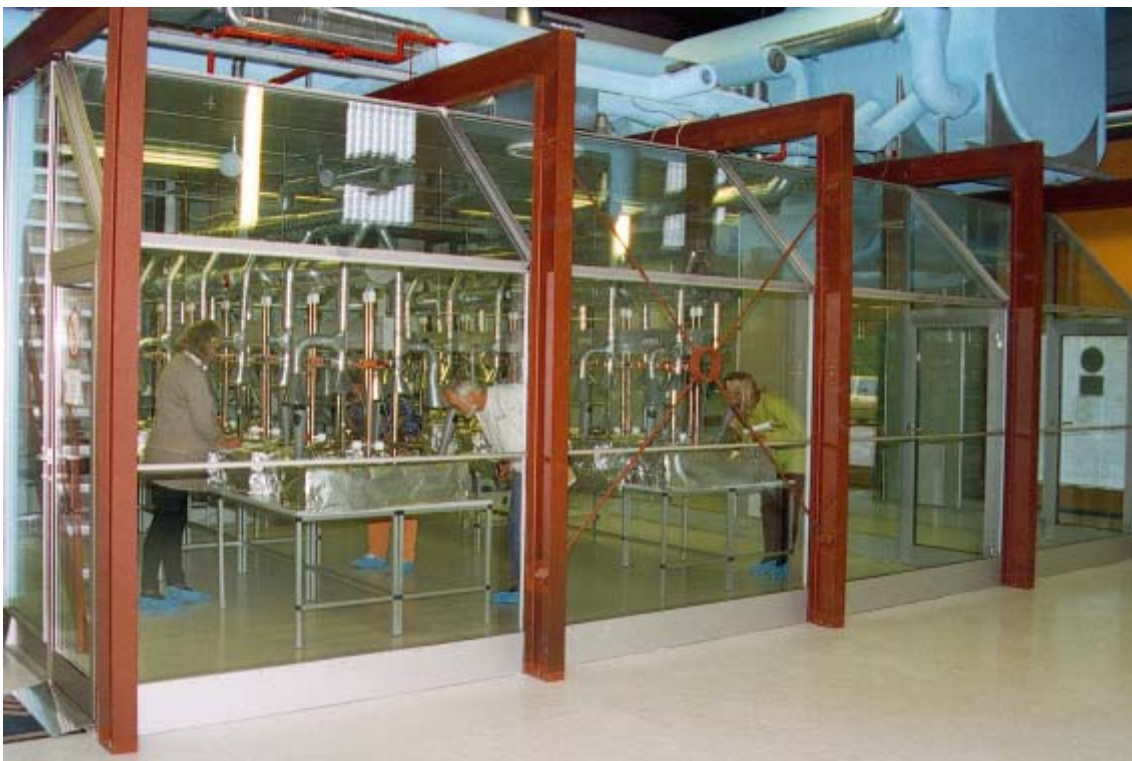
Figure 1. The exterior of the air quality laboratory with the main room to the left and the ante-room to the right. The ventilation and air-conditioning system and the duct-work are located at the roof of the laboratory.
